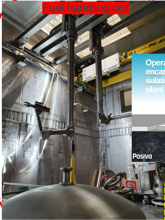
Manipulator for maintenance work at the fuel handling cell
