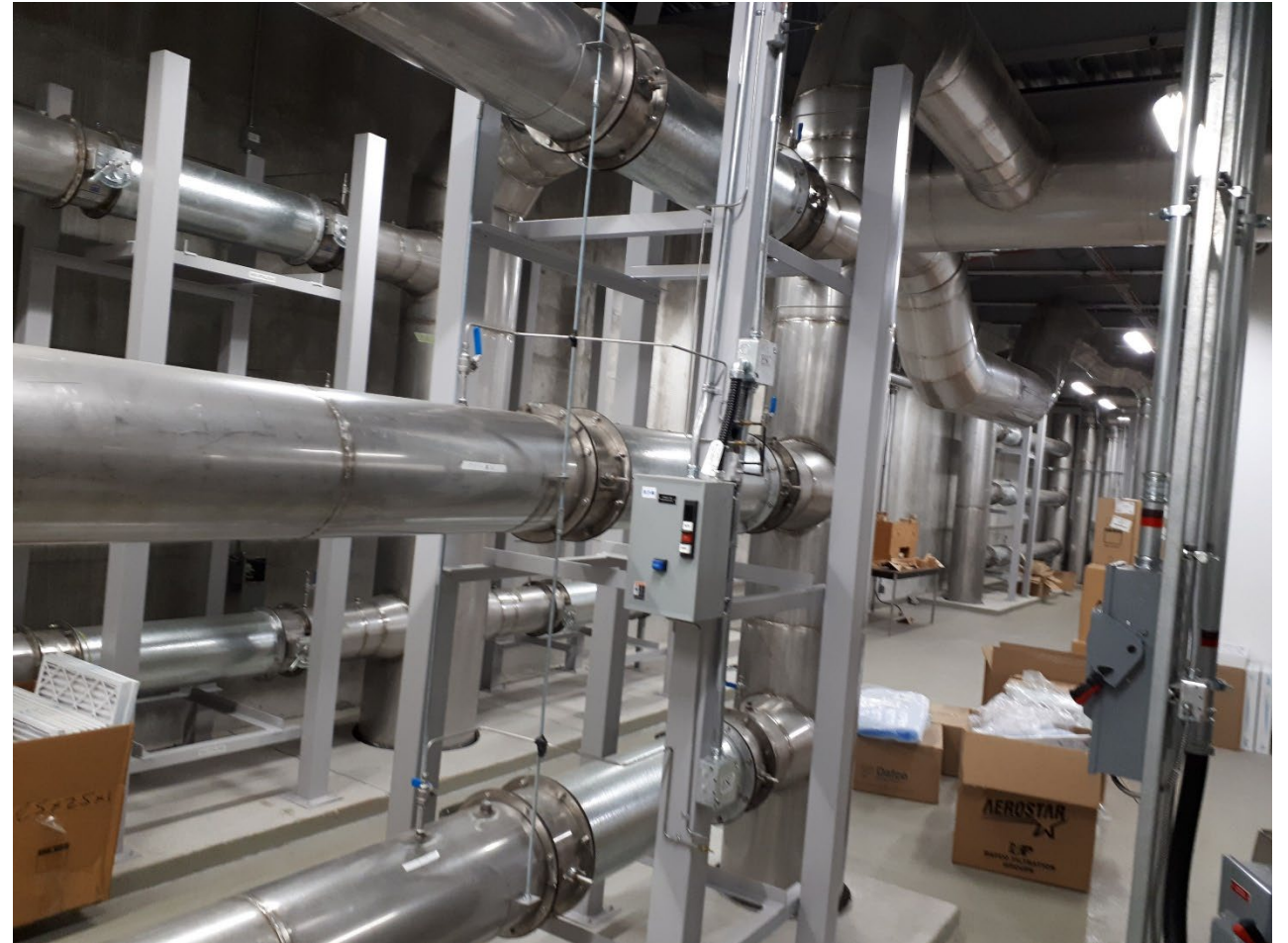
ARIEL Nuclear Ventilation Service Room at TRIUMF Image used with permission
