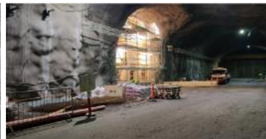
Technical rooms –437 m
