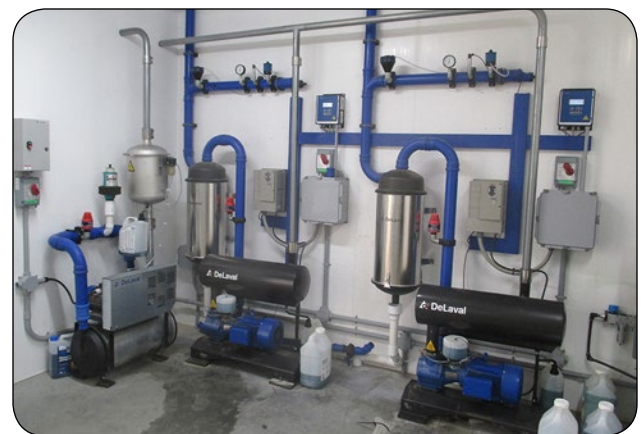
Figure 1. Equipment room free of clutter, dust and debris. Source: Heartland Farm Mutual, Ontario.
