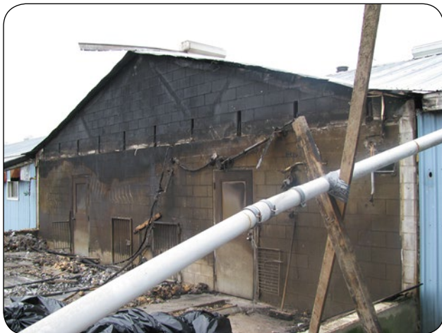
Figure 7. Example of an intact fire separation that did its job and prevented fire from spreading through the barn. Source: R. Drysdale, Farm Mutual Reinsurance Plan.
