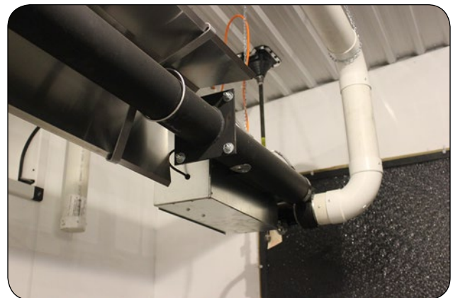
Figure 8. Radiant tube heater suspended in barn.
