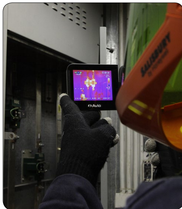
Figure 5. Inspection of electrical equipment by insurance company. Source: Heartland Farm Mutual, Ontario.
