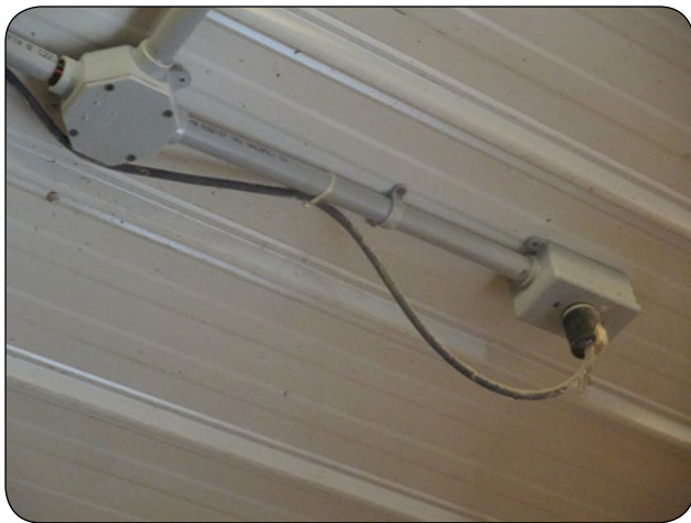
Figure 2. Temporary electrical equipment plugged into receptacle in livestock area. Source: Heartland Farm Mutual, Ontario.
